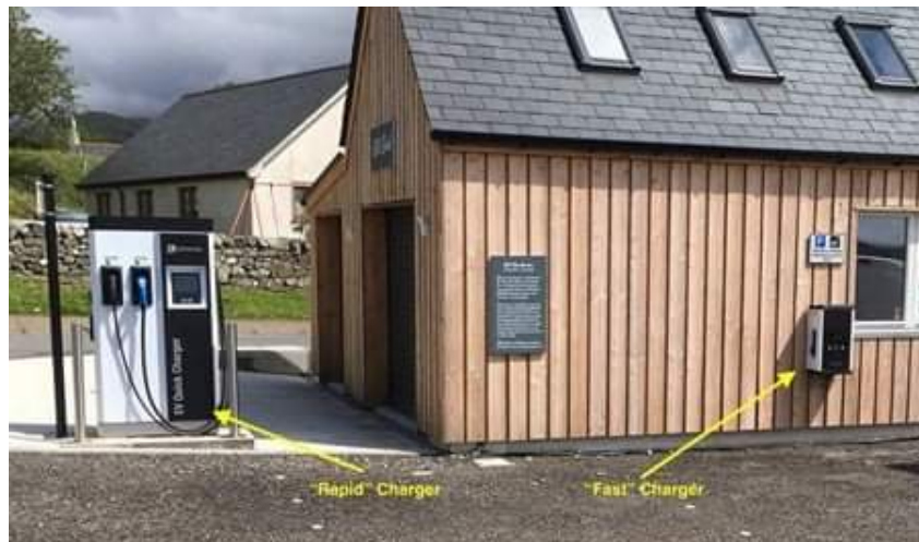
Figure 7: Photo of the EV chargers located at the LSIC
